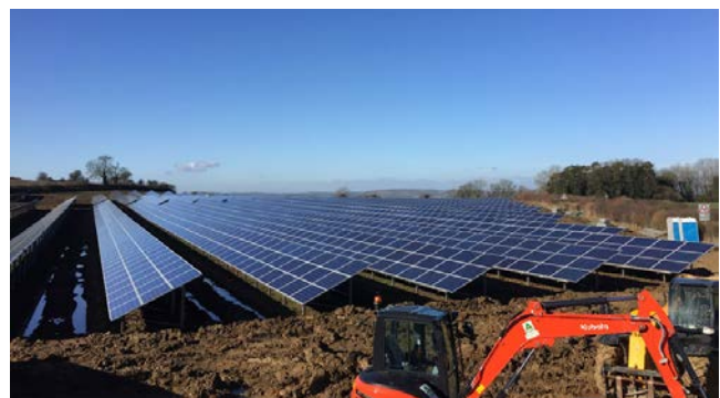
A 2.34MW solar array at Wilmington Farm, installed by Bath and West Community Energy. Photo: Bath and West Community Energy. http://www.bwce.coop/projects/wilmington-farm/
